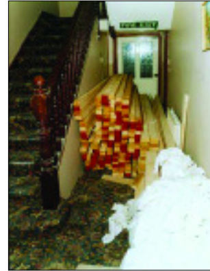
Figure 9: A blocked corridor with incorrect signage
